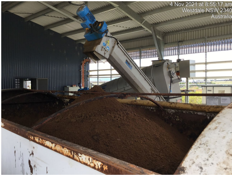
Photo 5: Solid by-products within the wastewater treatment plant
