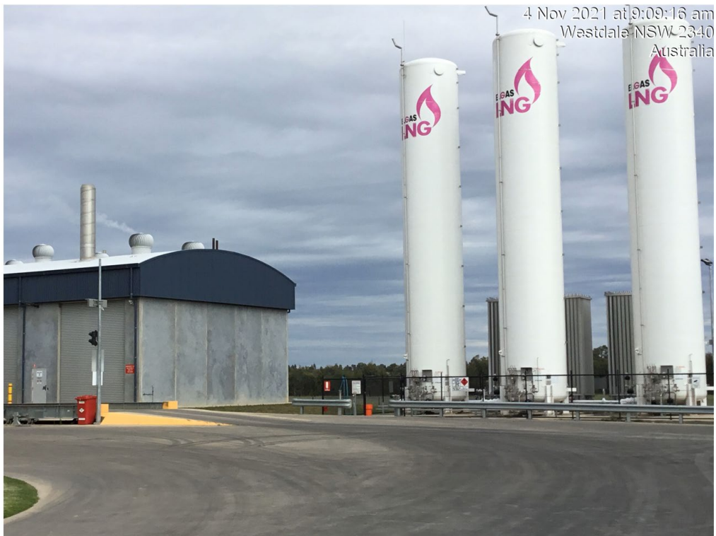
Photo 1: Northwest corner of the main plant showing the LNG storage tanks
